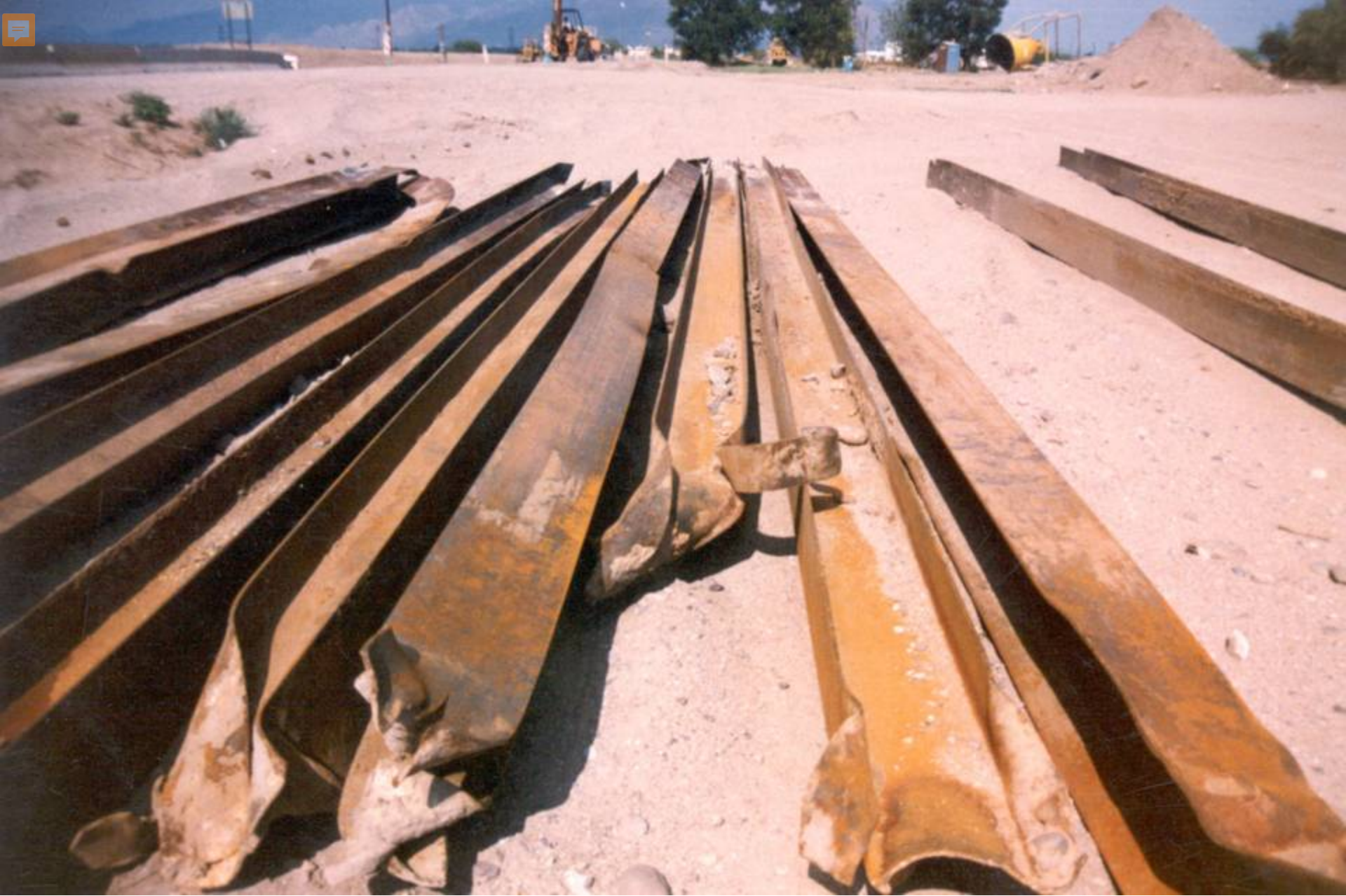
Damaged H-Beams after extraction.
